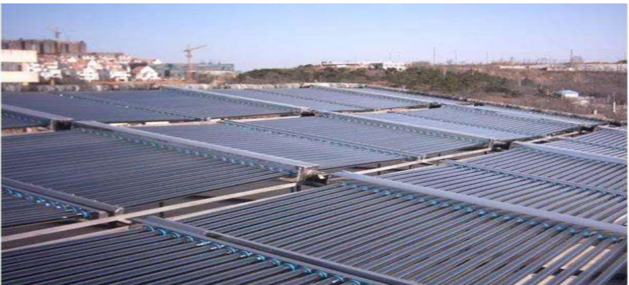
Figure 5.4.1: Solar Heater Field System
